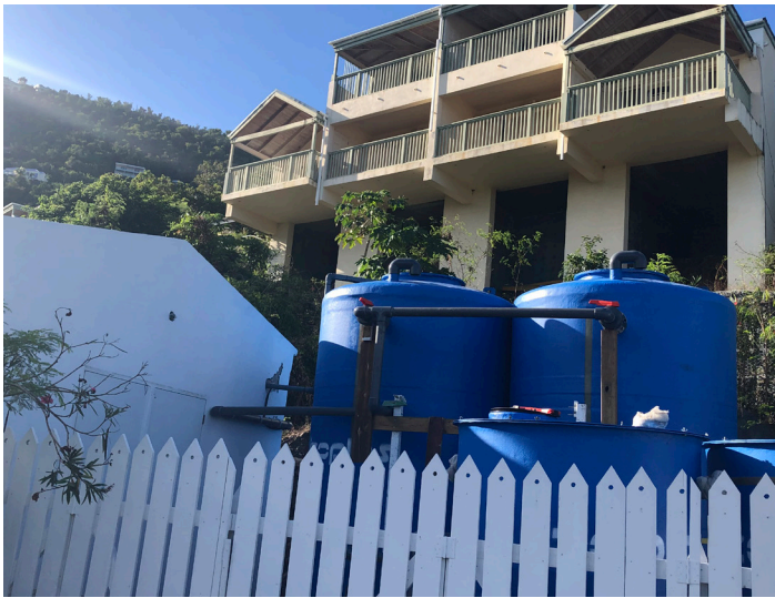
The Membrane BioReactor (MBR) tanks installed at the Long Bay Hotel & Resort provide compact, reuse-quality wastewater treatment in a coastal setting.
